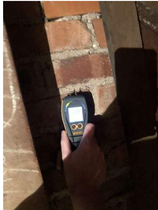
Party wall damp check.
