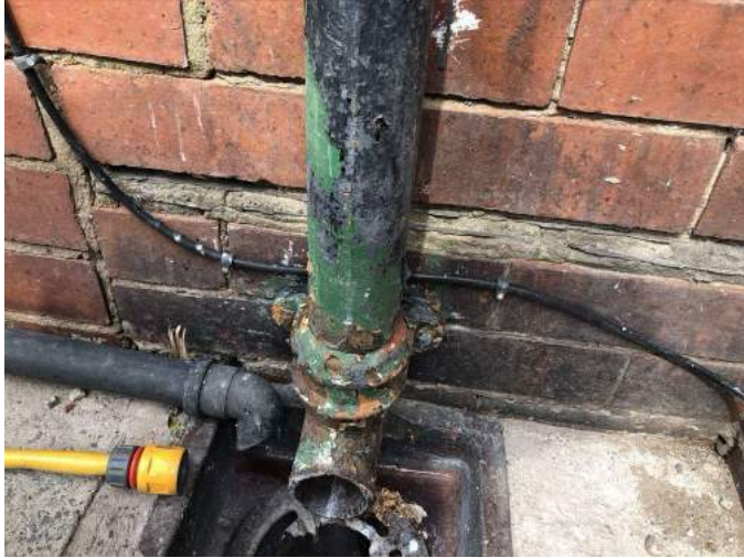
Corroded down pipe.
