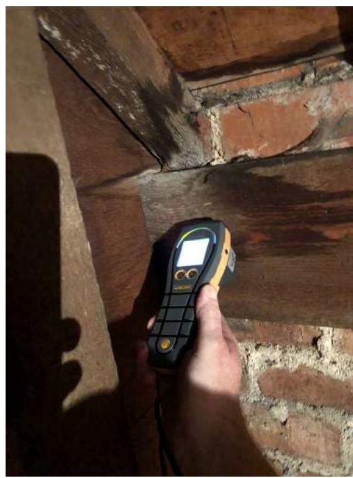
Purlin stain damp check.
