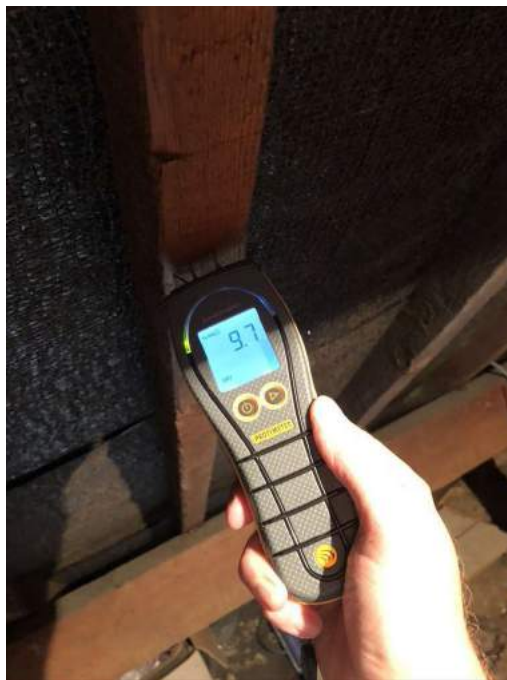
Rafter damp check.
