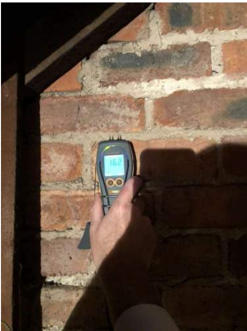
Party wall damp check.
