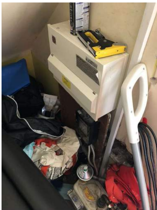
RCD fuse board.
