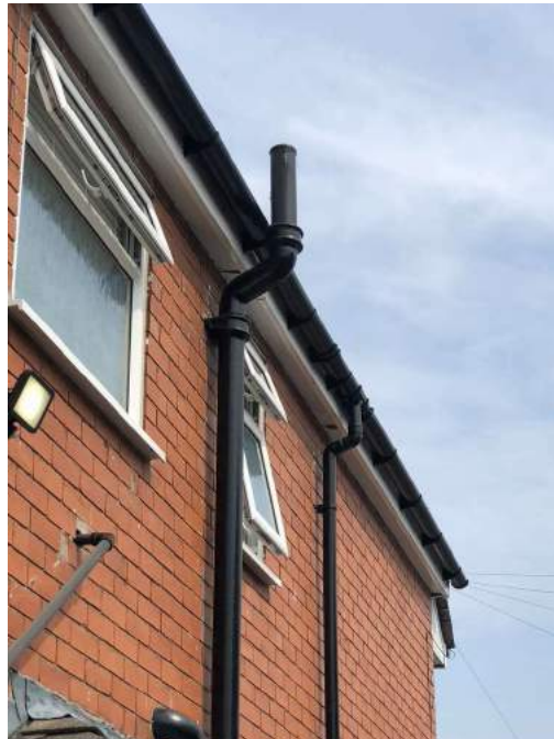
Soil pipe with no cage on top.
