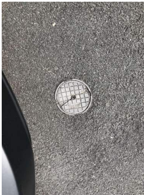
Damaged water meter cover.
