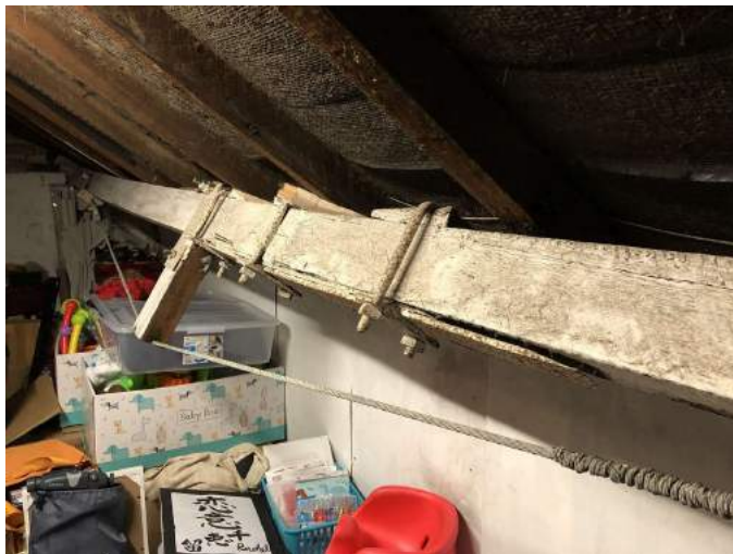
Bowed purlin, packers and brackets.
