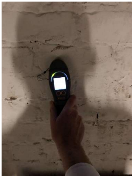
Party wall damp check.
