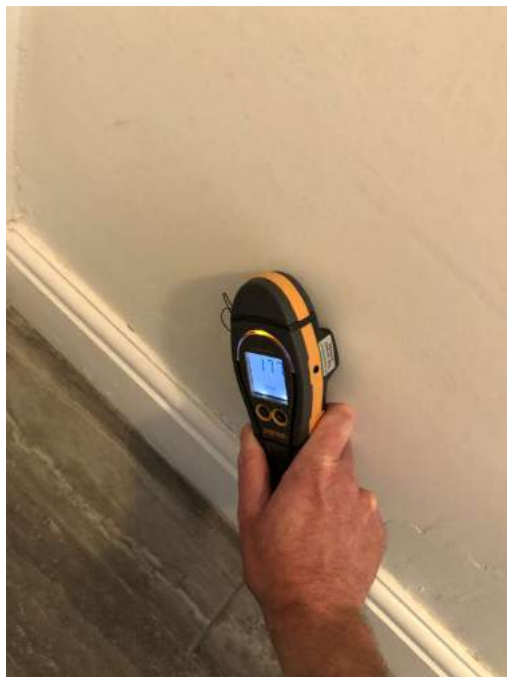
Internal damp check. Medium reading.
