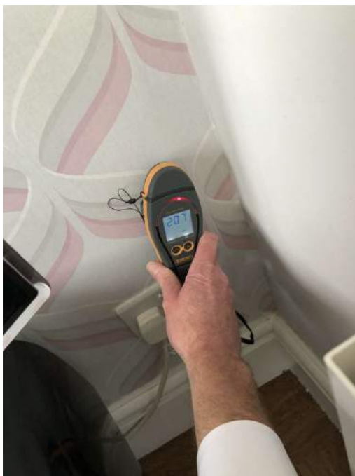
Internal damp check. High reading.
