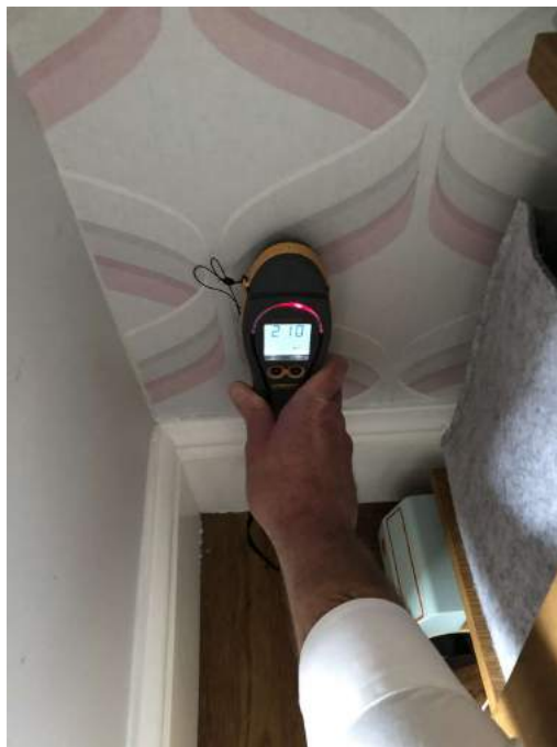
Internal damp check. High reading.
