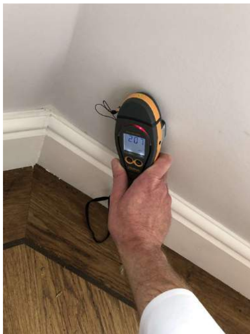
Internal damp check. High reading.
