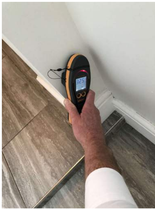
Internal damp check. High reading.
