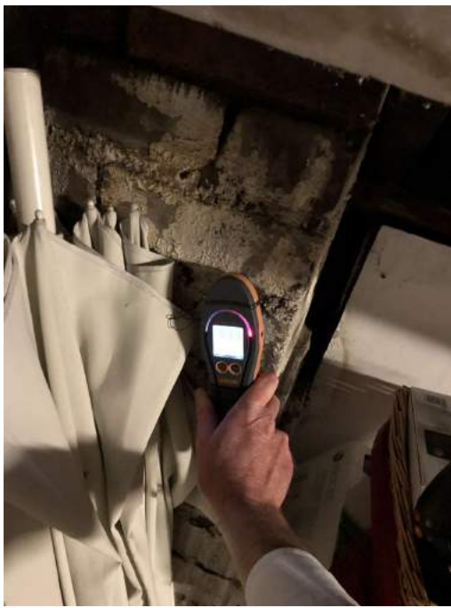
Chimney stack damp check. High reading.
