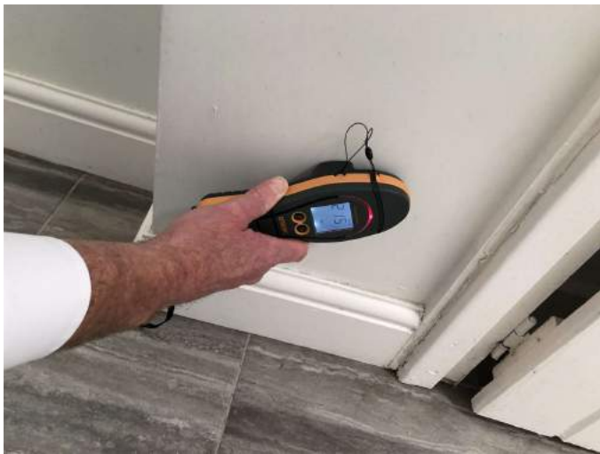
Internal damp check. High reading.
