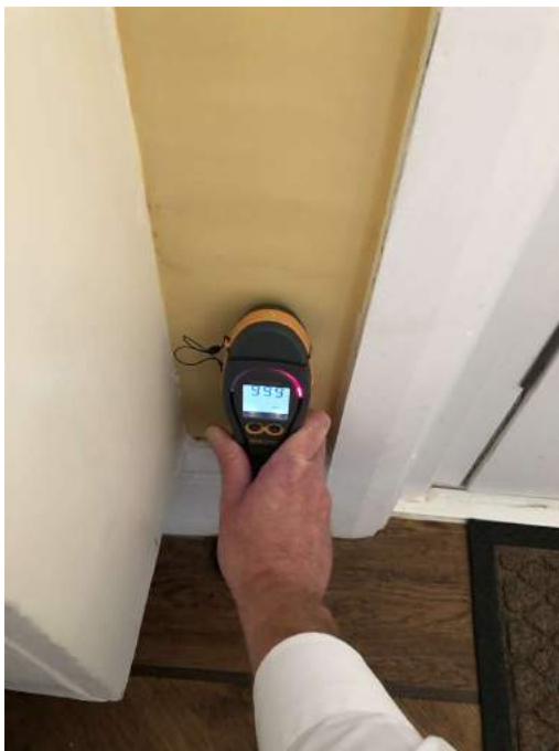
Internal damp check. High reading.
