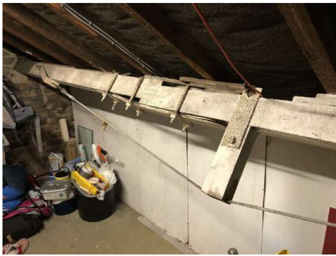
Bowed purlin showing where part of the roof structure has been removed.
