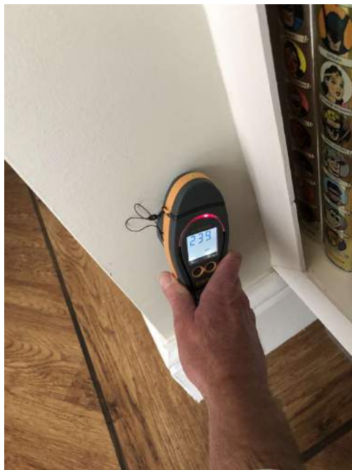
Internal damp check. High reading.
