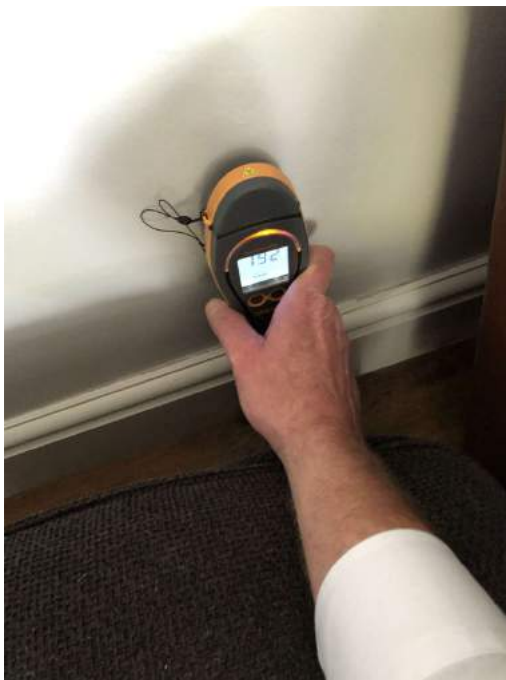
Internal damp check. Medium reading.
