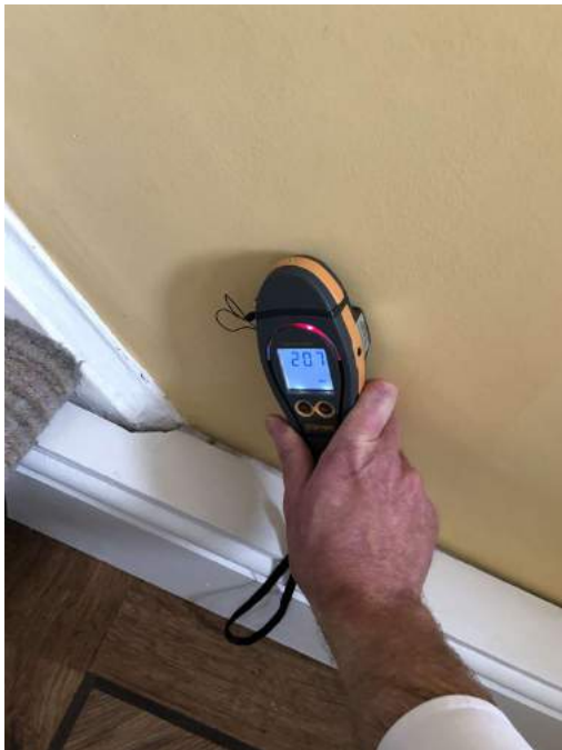
Internal damp check. High reading.
