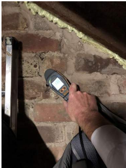
Party wall damp check.
