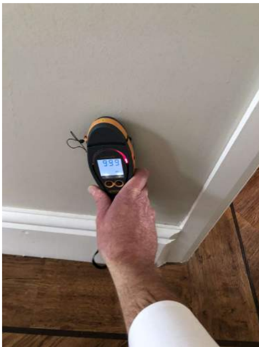
Internal damp check. High reading.
