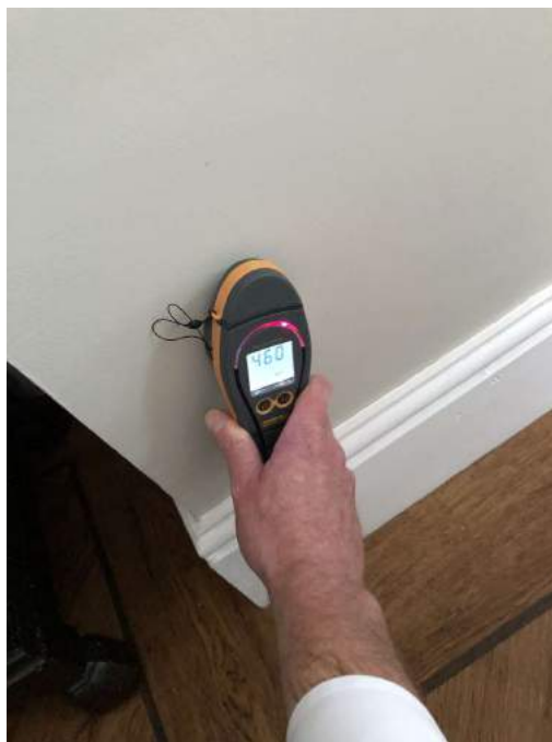
Internal damp check. High reading.
