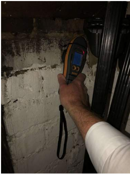
Chimney stack damp check. High reading.
