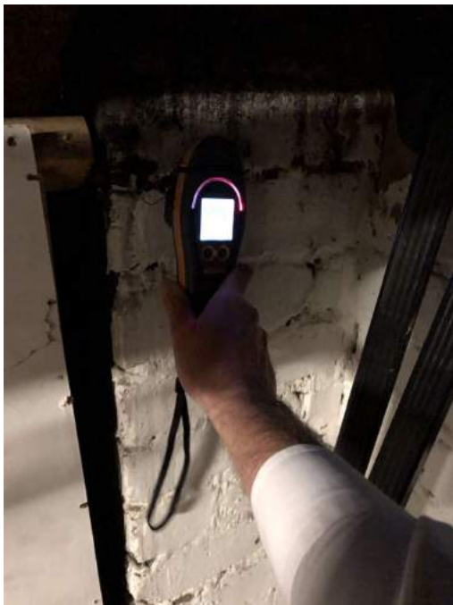
Chimney stack damp check. High reading.
