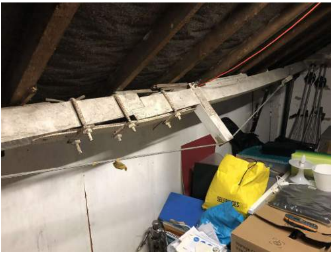
Bowed purlin, brackets and packers.
