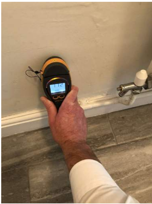
Internal damp check. Medium reading.
