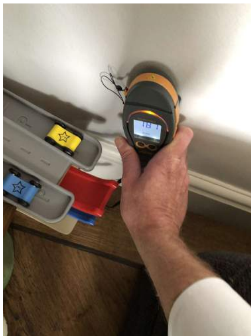
Internal damp check. Medium reading.
