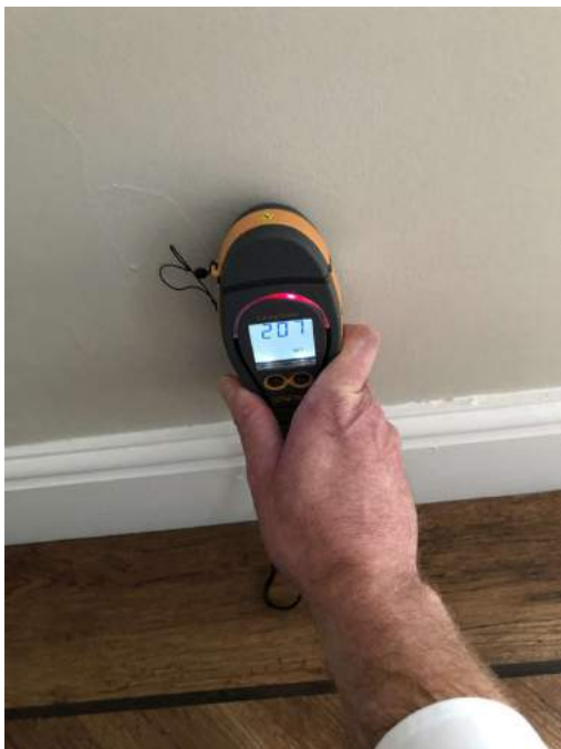
Internal damp check. High reading.
