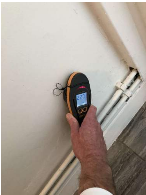
Internal damp check. High reading.
