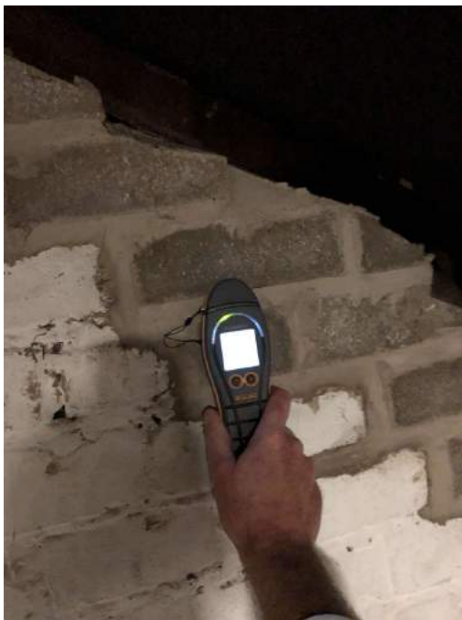
Party wall damp check.
