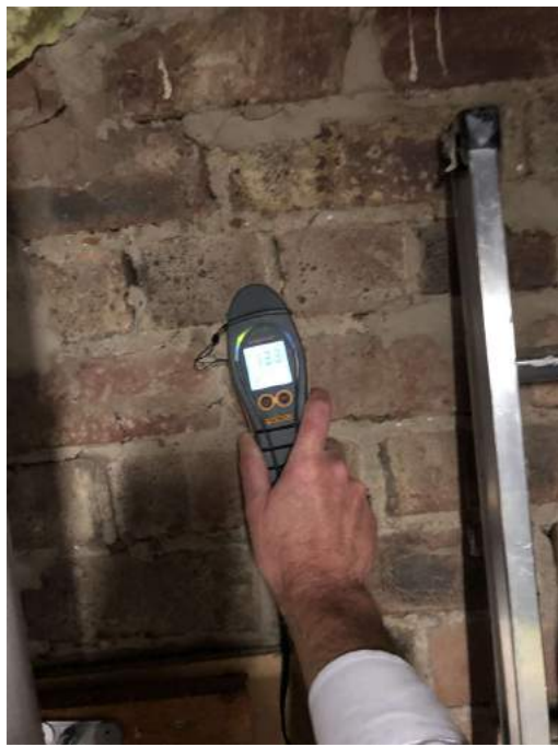
Party wall damp check.
