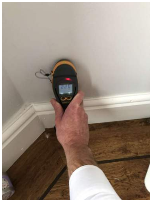
Internal damp check. High reading.
