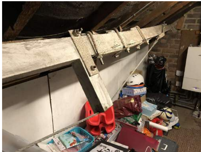
Bowed purlin showing where part of roof structure has been removed.
