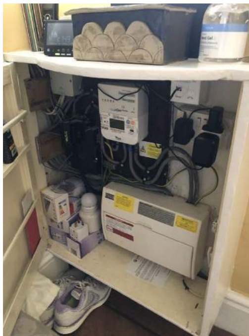
Electric meter and RCD consumer unit.
