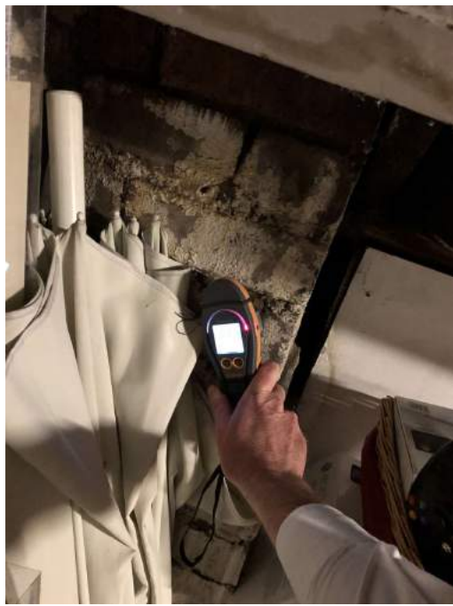
Chimney stack damp check. High reading.
