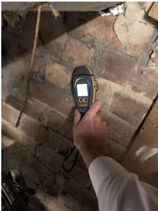
Party wall damp check.
