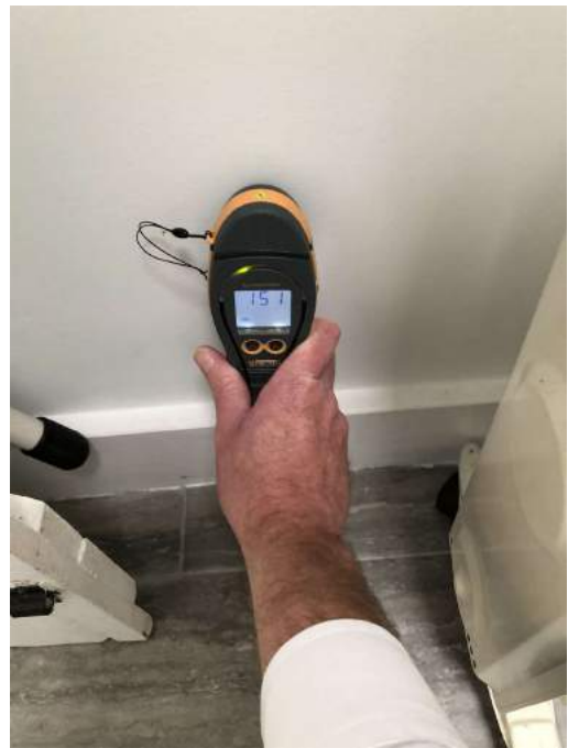
Internal damp check. Low reading.
