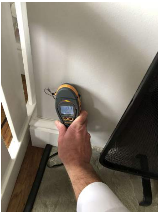
Internal damp check. Medium reading.
