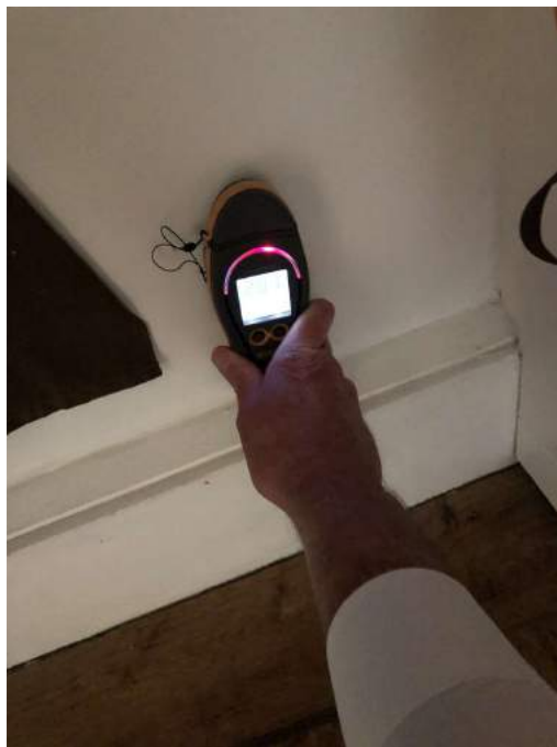
Internal damp check. High reading.
