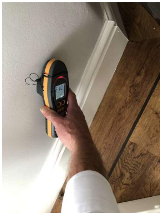
Internal damp check. High reading.
