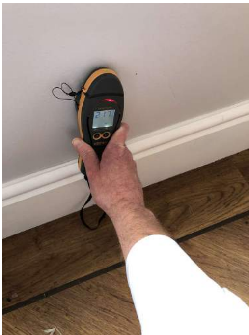
Internal damp check. High reading.
