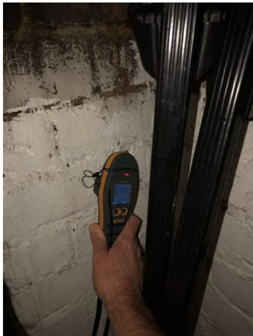
Chimney stack damp check. High reading.
