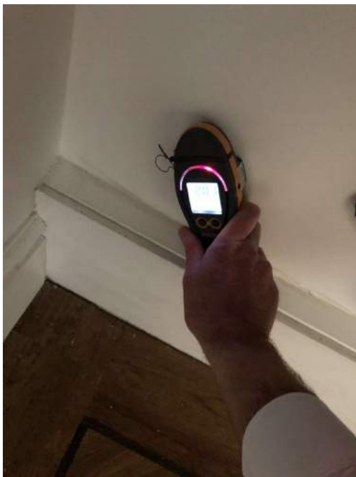
Internal damp check. High reading.
