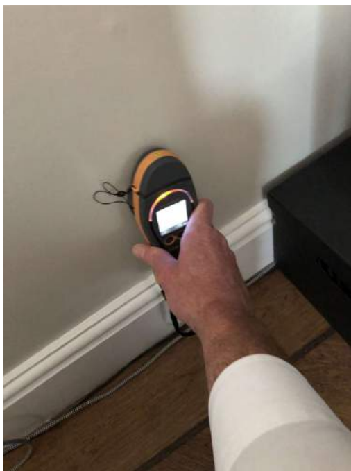
Internal damp check. Medium reading.
