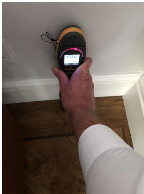
Internal damp check. High reading.
