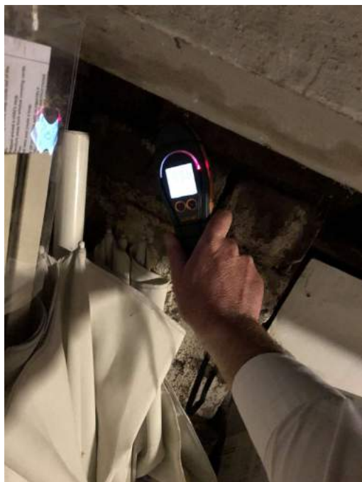
Chimney stack damp check. High reading.
