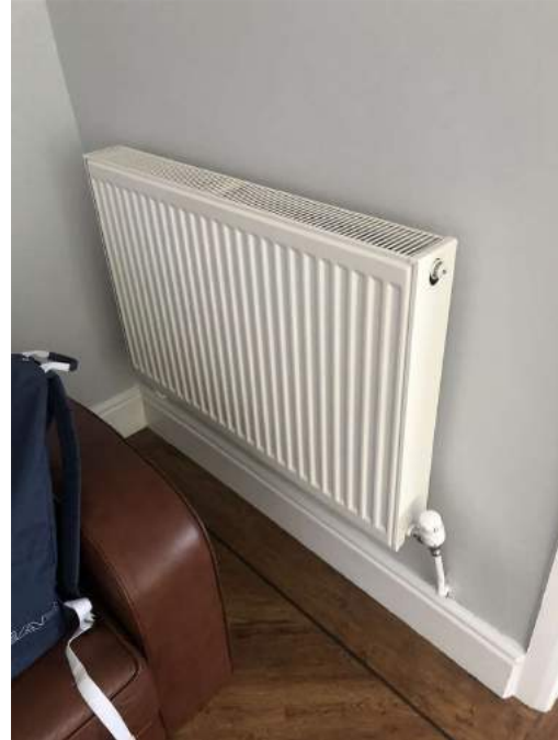
Radiator and TRV.
