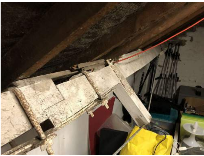
Bowed purlin, packers and brackets.
