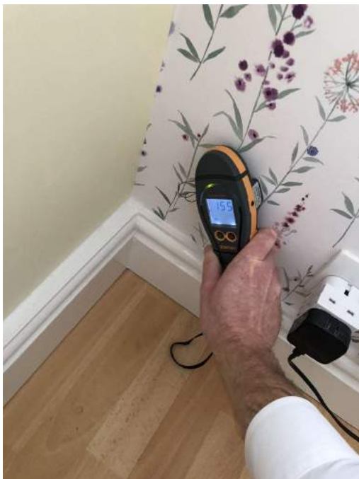
Internal wall damp check.
