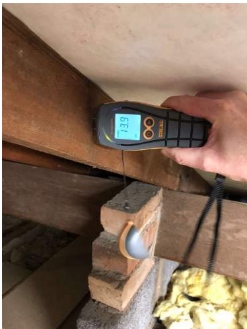
Rafter damp check.
