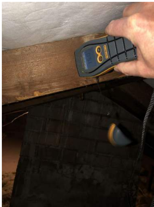
Rafter damp check.
