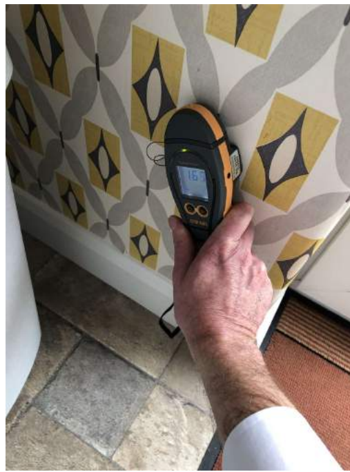
Internal wall damp check.
