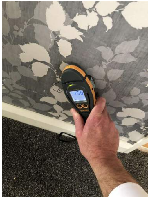
Internal wall damp check.
