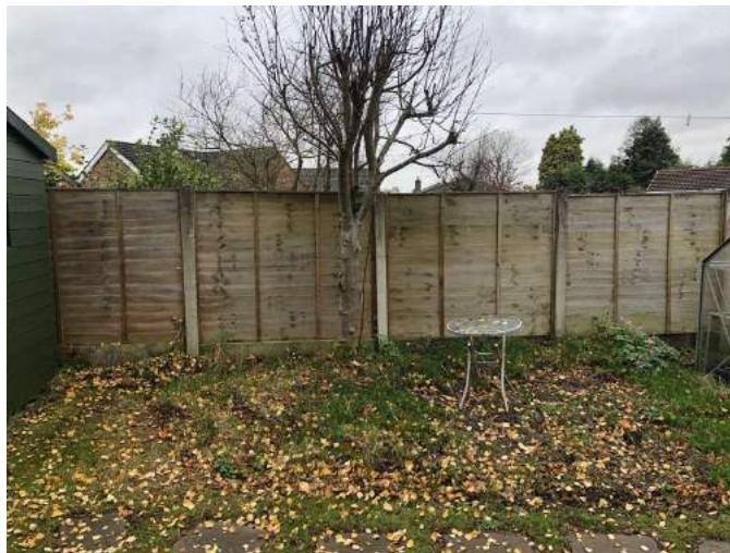
Timber fence panels.
