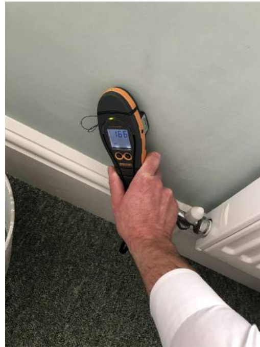
Internal wall damp check.
