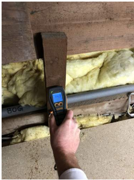
Hanger damp check.
