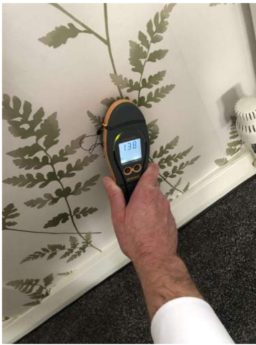
Internal wall damp check.
