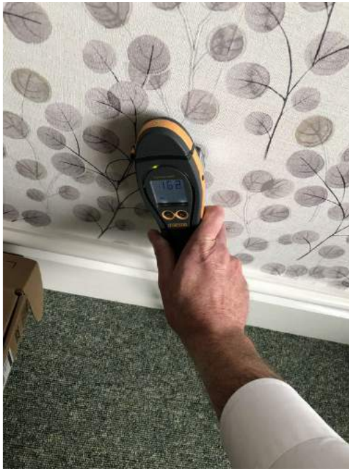
Internal wall damp check.
