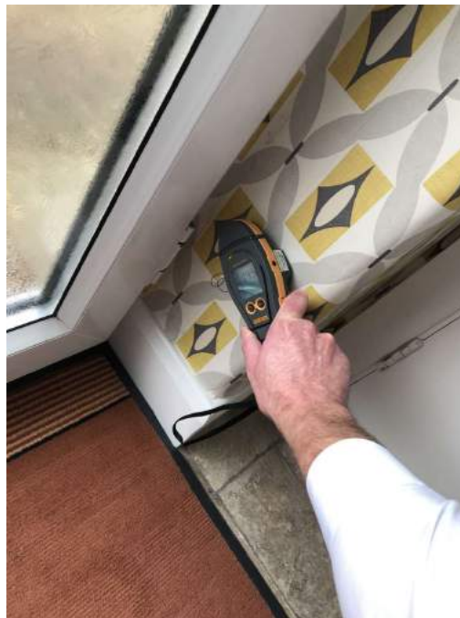
Internal door reveal damp check.
