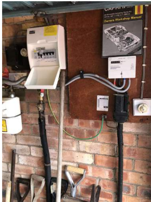
RCD Consumer unit and electric meter.
