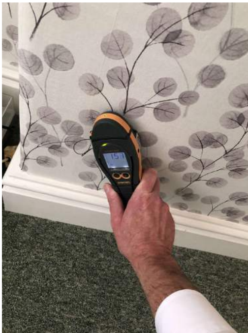
Internal wall damp check.
