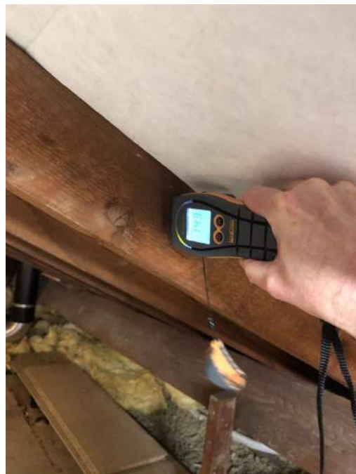
Rafter damp check.
