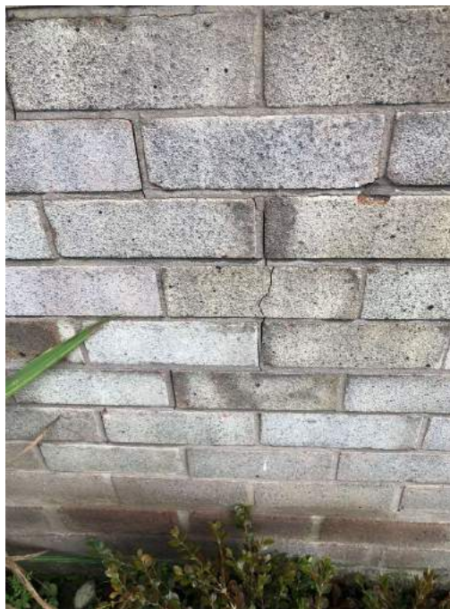
Crack to brick in front wall below window.
