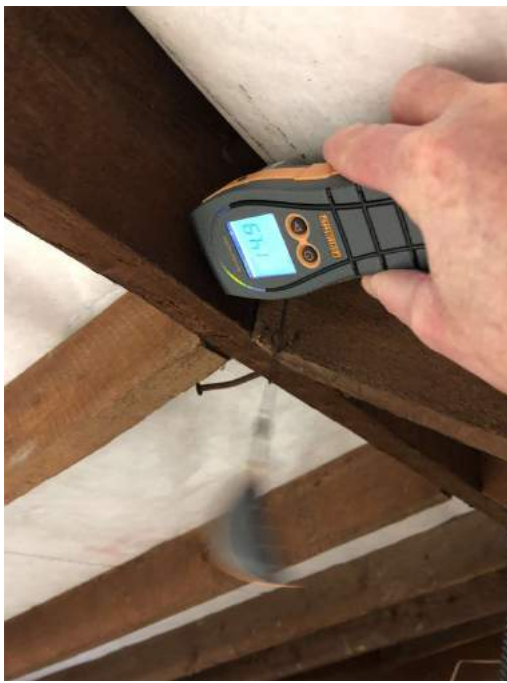
Rafter damp check.
