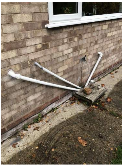
Kitchen waste pipes.
