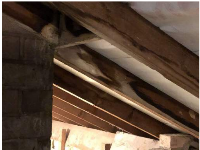
Staining to rafter next to chimney stack.
