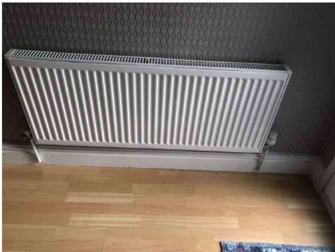
Radiator and TRV.
