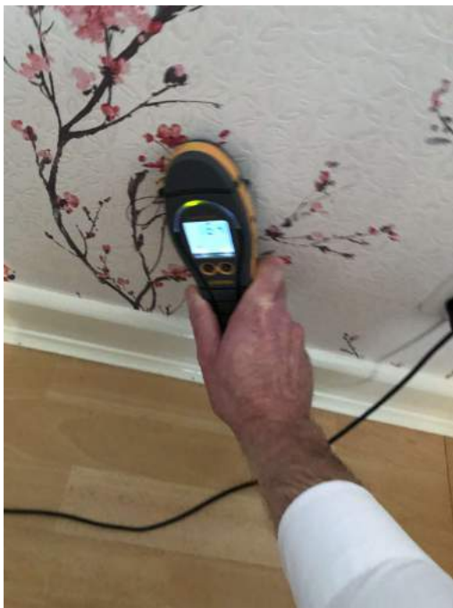
Internal wall damp check.
