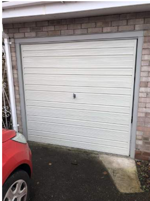
Garage up and over door.
