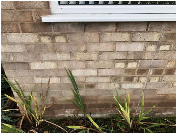
Cracking to front wall below window.
