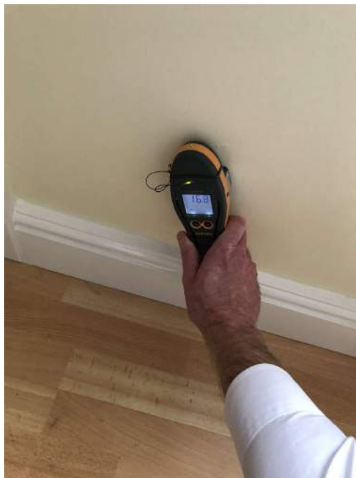
Internal wall damp check.
