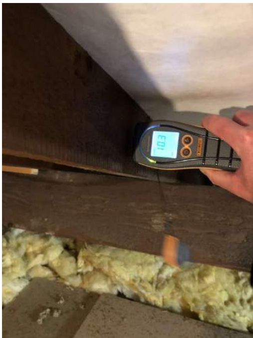
Rafter damp check.
