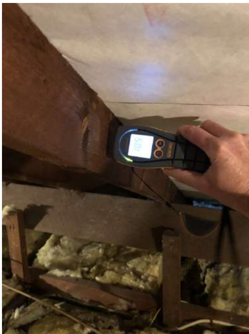
Rafter damp check.
