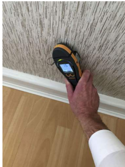
Internal wall damp check.
