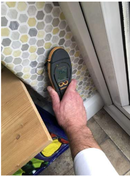
Internal door reveal damp check.
