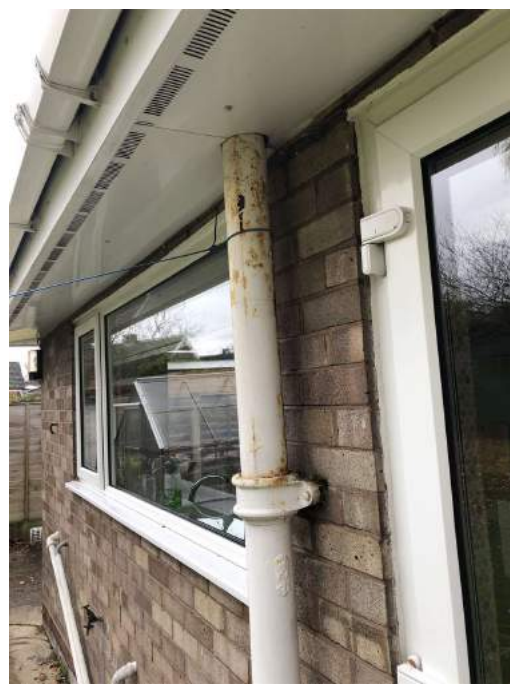
Rear drainage ventilation pipe.
