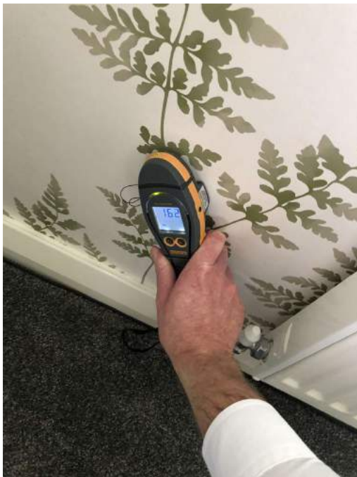
Internal wall damp check.
