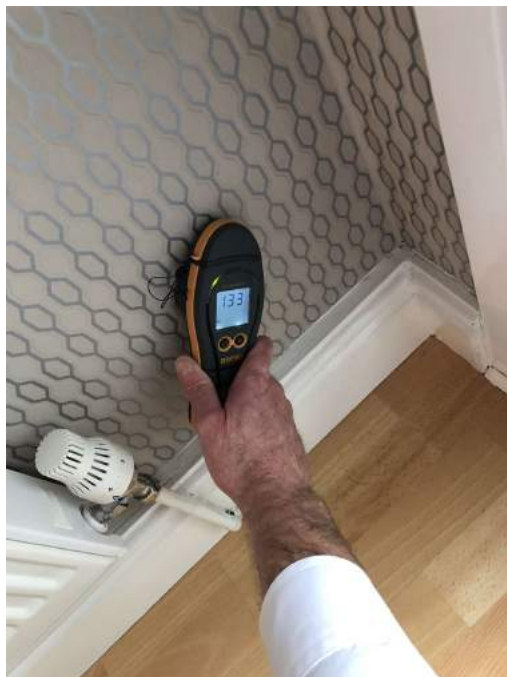
Internal wall damp check.
